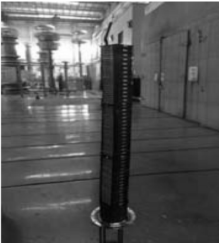
图8 CVT B相中节电容分压器电容心子 Fig. 8 Capacitor core of middle capacitor voltage divider in phase B of CVT
